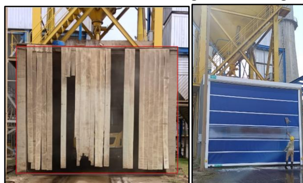
Figure 8. Fly ash silo unloading area before (left) and after (right) installation
