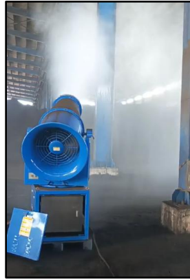
Figure 1. Fog cannon installation in the coal shed area
